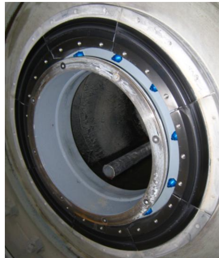
Fig. 16. Picture of the stator containing the flushing nozzles
